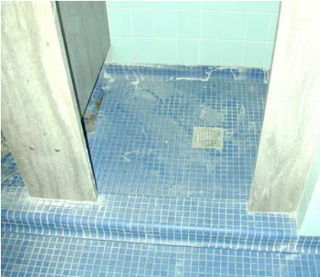
EXISTING LEAKING SHOWERS
